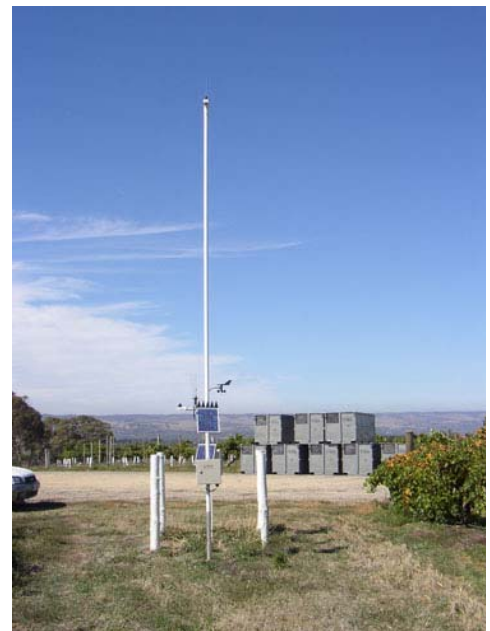
BRL Hardy Wines – South Australia.. Soil moisture monitoring system.
